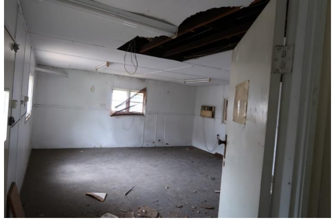
Partially collapsed ceiling
