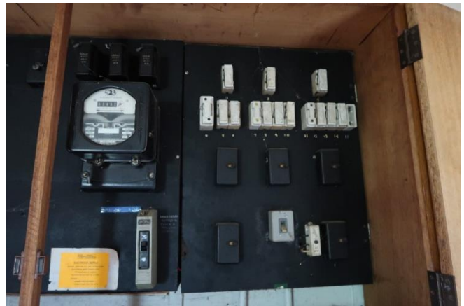
Main distribution board
