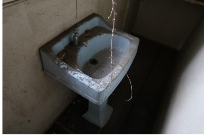
Amenities fixtures in poor condition
