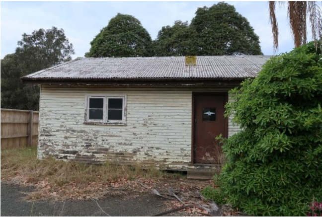
Asbestos roof sheeting and deteriorated cladding
