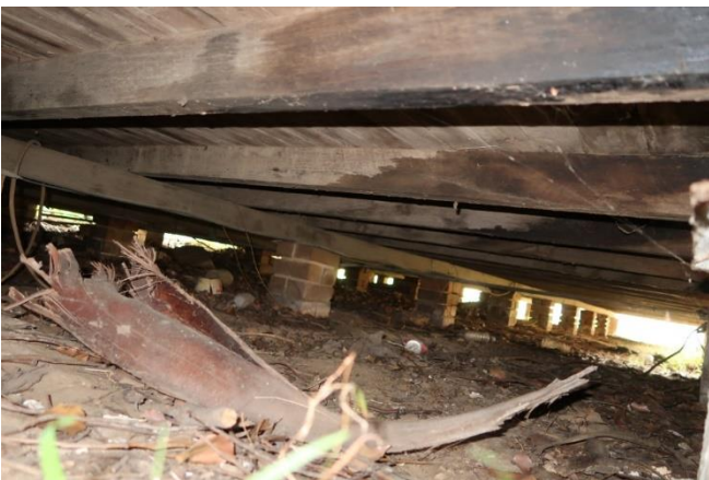
Damp timbers to suspended floor structure
