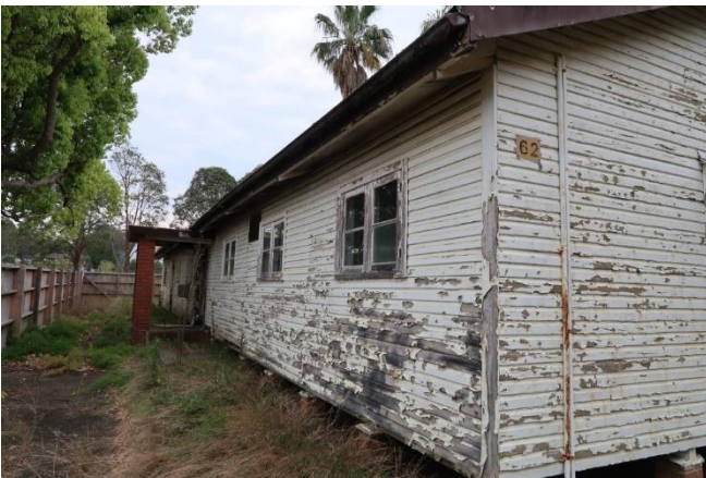
Building fabric in poor condition
