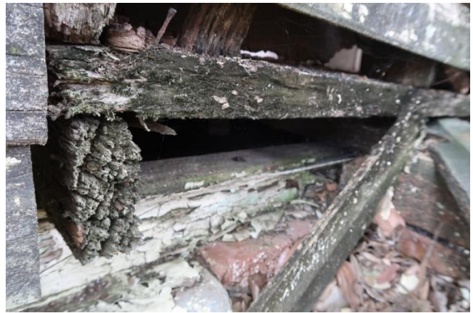
Rotted timber frame
