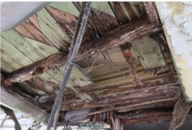
Rotted timber frame
