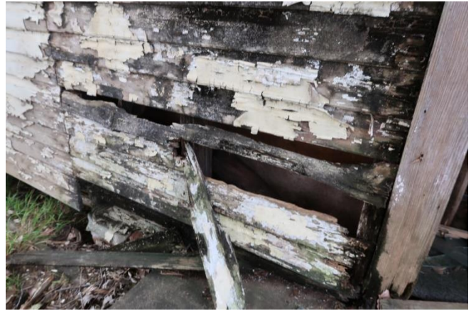
Rotted timber cladding
