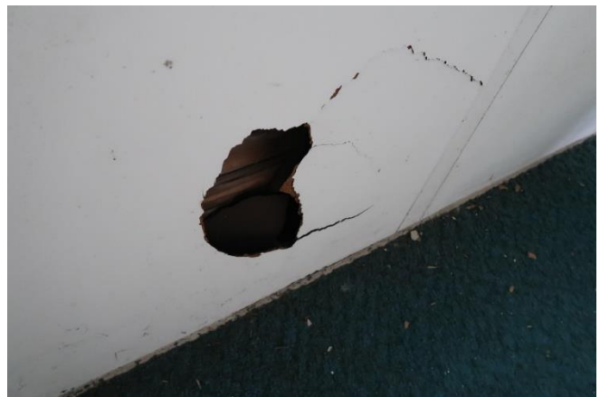
Impact damaged wall
