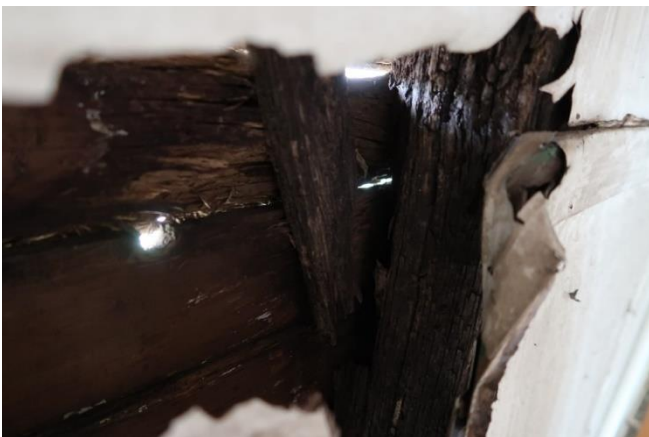
Rotted timber frame
