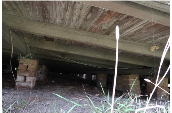
Deteriorated mortar beds and 'leaning' pier
