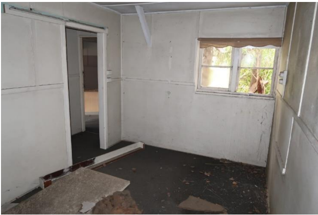
Interior finishes in poor condition
