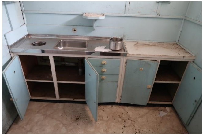
Kitchen cabinetry in poor condition
