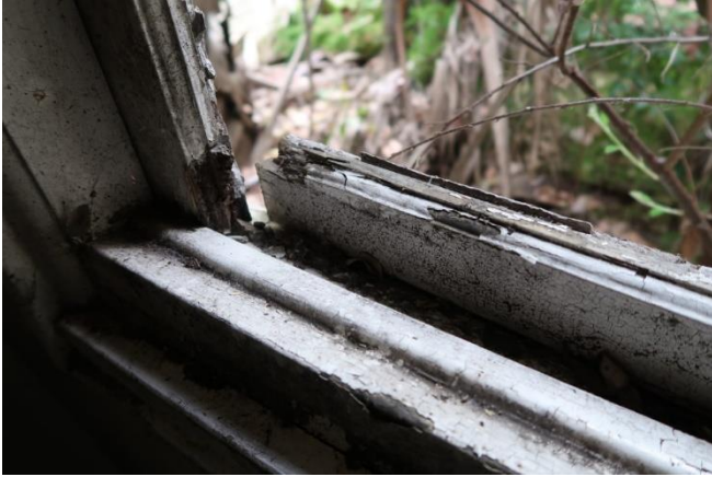
Window frame in poor condition
