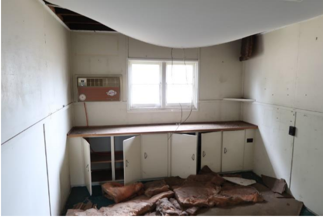
Partially collapsed ceiling
