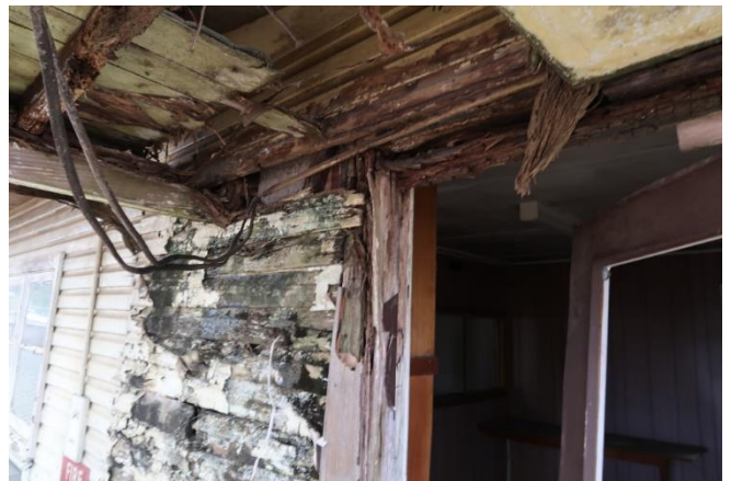
Rotted timber frame
