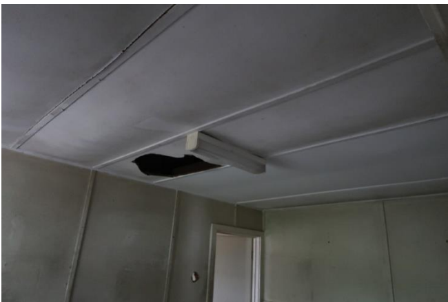
Water damaged ceiling
