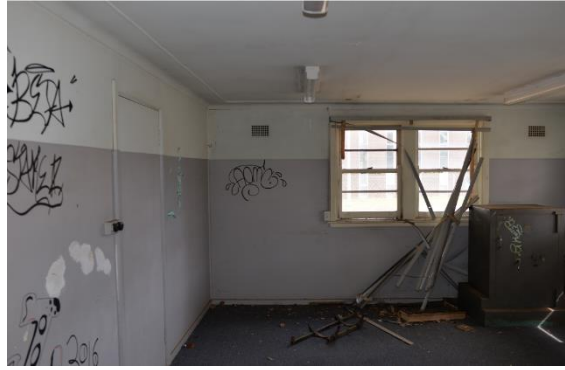
Figure 18. Vandalism and dilapidated window in southern wing of the building.
