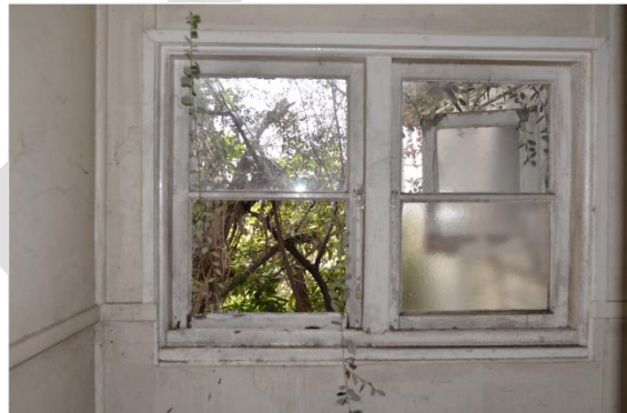
Figure 20. Broken windowpane with overgrown vegetation.
