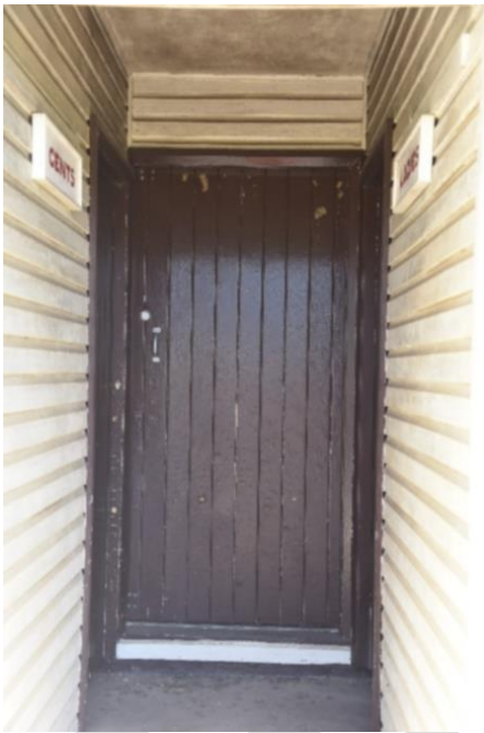
Figure 13. Original entry beneath the awning on the building's east elevation, with lavatory signage.
