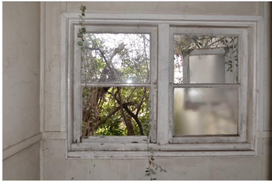
Figure 16. Broken windowpane with outdoor vegetation creeping in.
