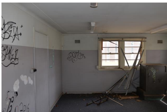
Figure 14. Vandalism and dilapidating window, southern wing.
